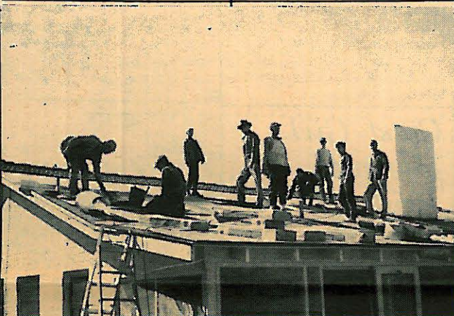
Men of the First Baptist Church of the Willows spend their Saturdays on the church. Here they are putting on new roof. (Echo-Sun Photo)
